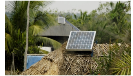
Solar Home System
