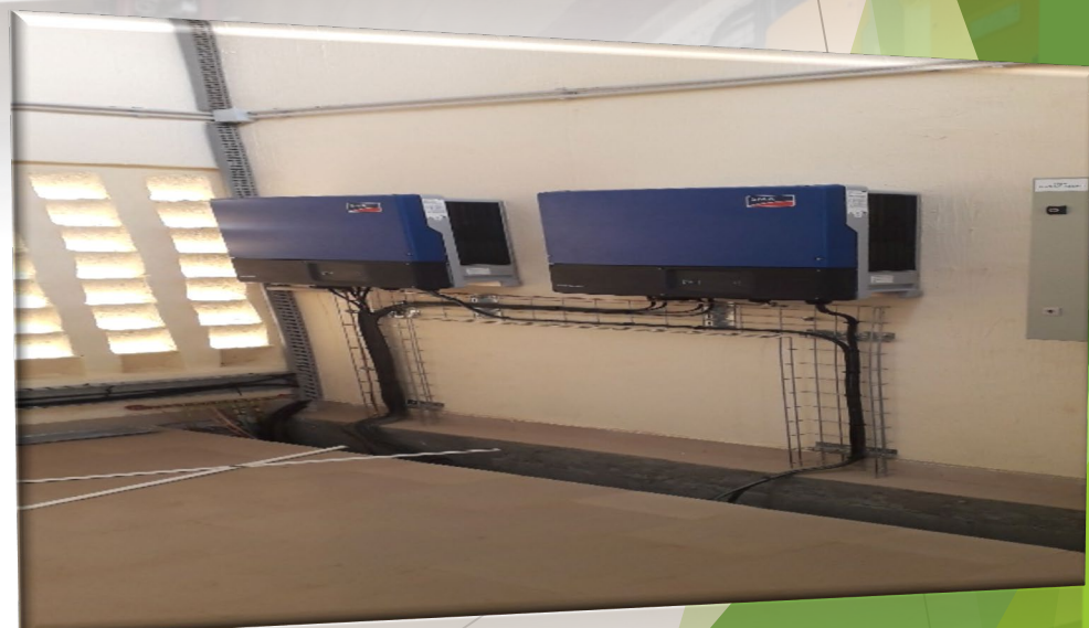
Battery and Network UPS Room
