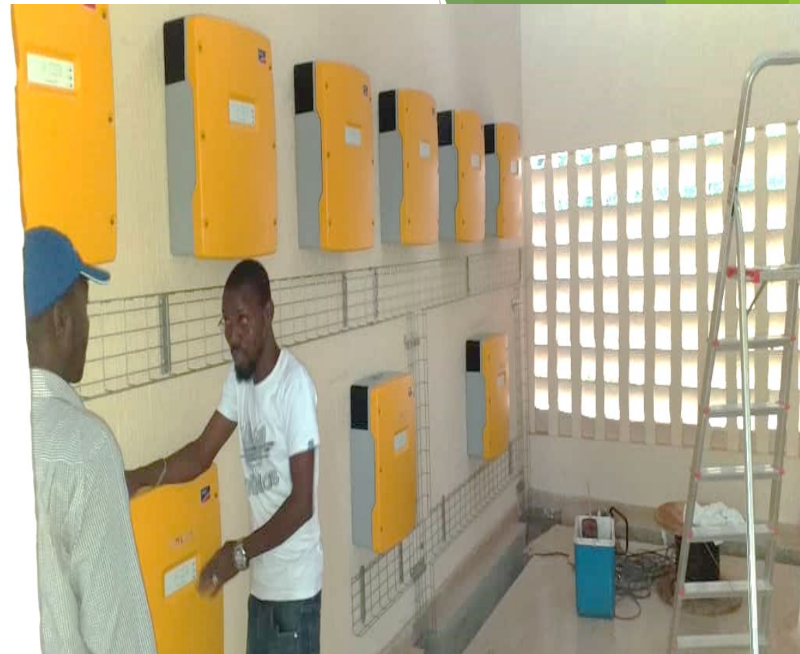
Garalo inverters room
