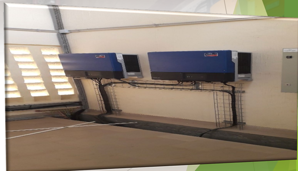
Battery and Network UPS Room
