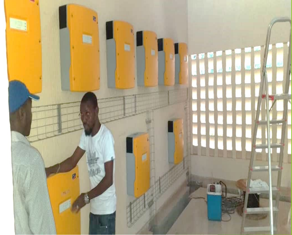
Garalo inverters room
