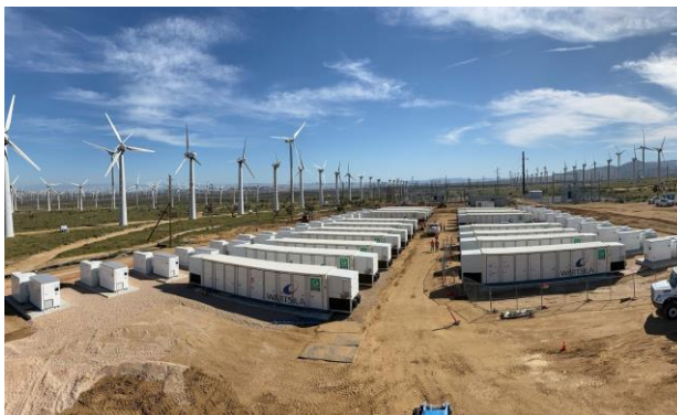
CA, USA 70MW/70MWh Renewables integration
